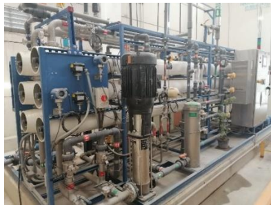
Wastewater treatment equipment at the Tlaxcala Plant (Mexico)
